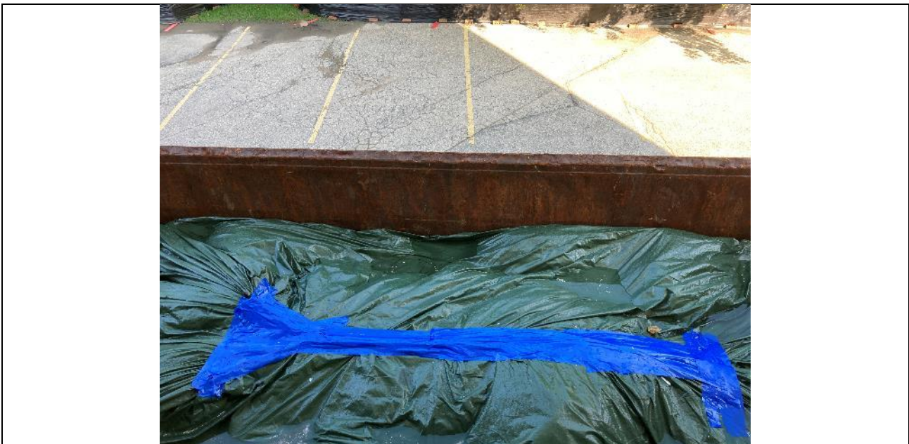
P6 – Asbestos Waste Bin
